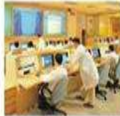
Control Center/Data Center
